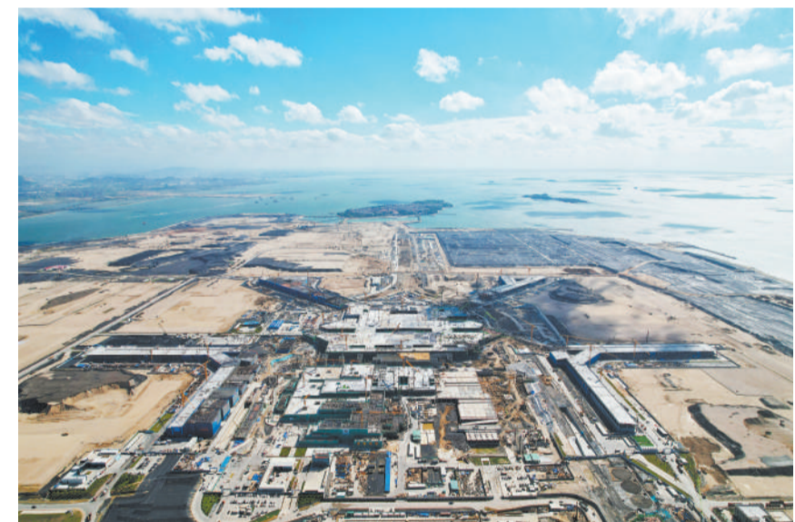
The construction of the Xiang'an International Airport on Dadeng Island in Xiamen, Fujian province, is progressing, with the main concrete structure of the terminal and the corridor completed on August 31 by China Construction Third Engineering Bureau Group. (PHOTO: LIN Hang)
