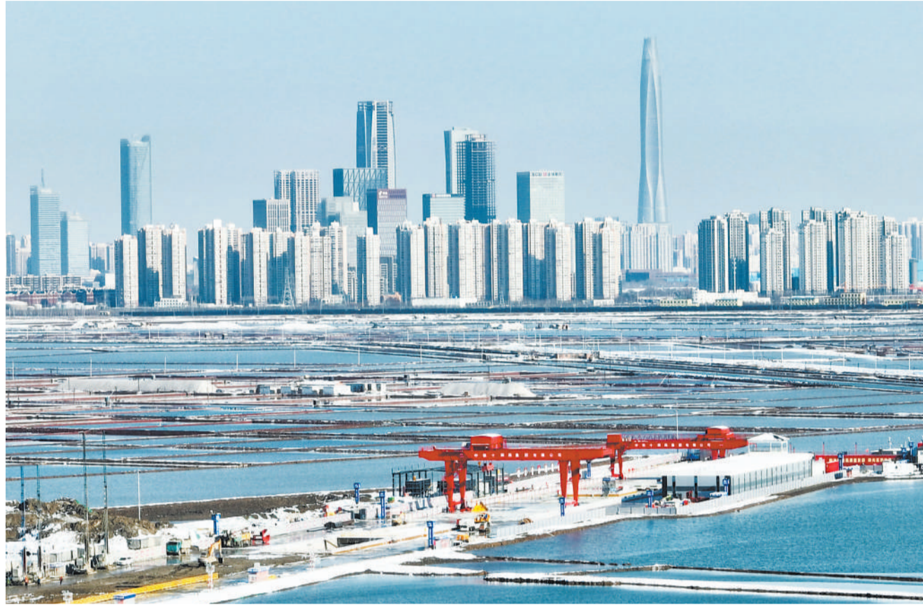
The Jingu Haihe Tunnel is the high-speed shield tunnel with the largest diameter and longest driving distance in the Beijing-Tianjin-Hebei region. (PHOTO: XINHUA)
